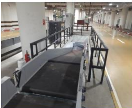
Baggage Breakup Area Conveyor Room
